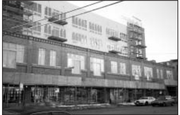
Typical of the new developments springing up on Morse Avenue are these 25 new luxury condo units being built on the 1200 block of Morse Avenue.
